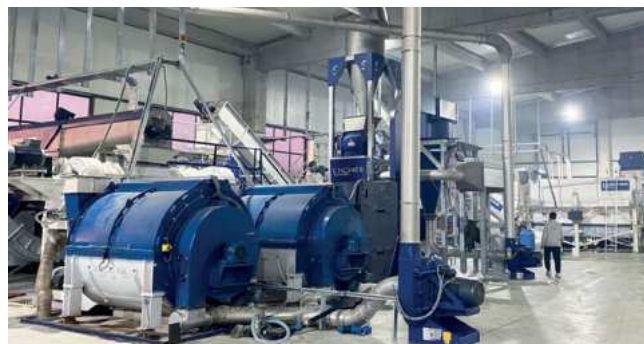
The washing line supplied by Lindner Washtech covers the entire recycling process at Plastika Kosovo – from shredding through washing and drying to extrusion (Images copyright © Lindner)
